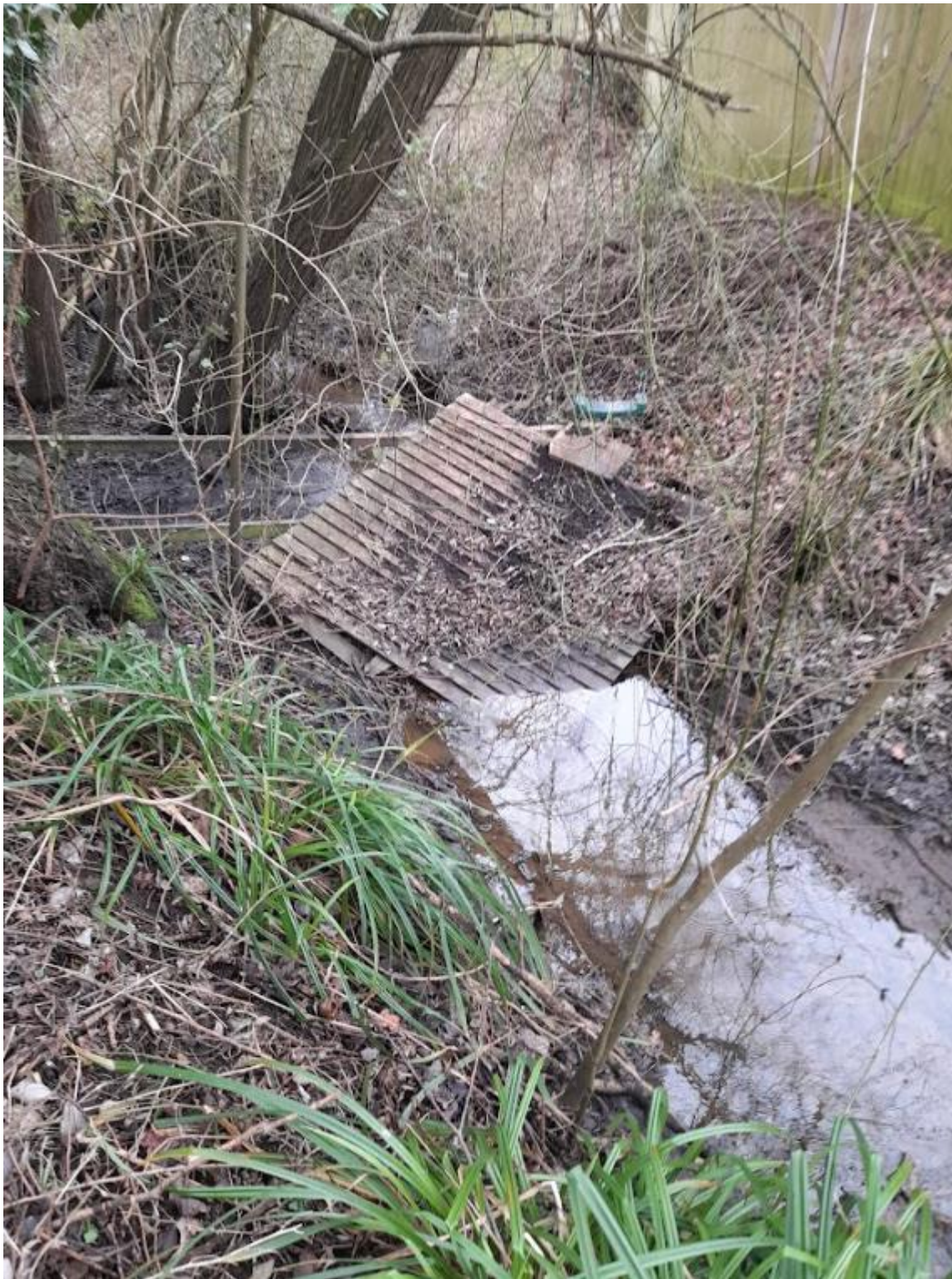
Photo 4. General waste, possible storm damage or fly tipping at a location in the drainage ditch. The direction of water flow is upper left to bottom right of the photograph.
